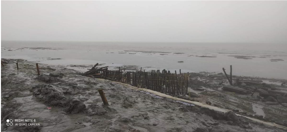
Fig.8: Demolition of earthen embankments which was covered with Geojute in Mousuni island, Baliara block. Source: Captured by author, 25 th august,2023
